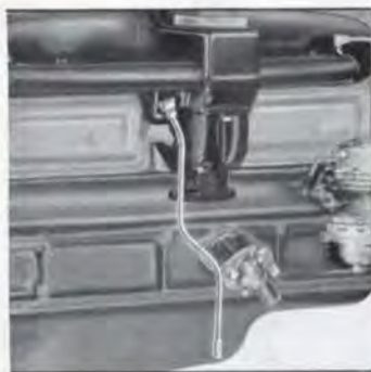
Condensation Drain Pipe
